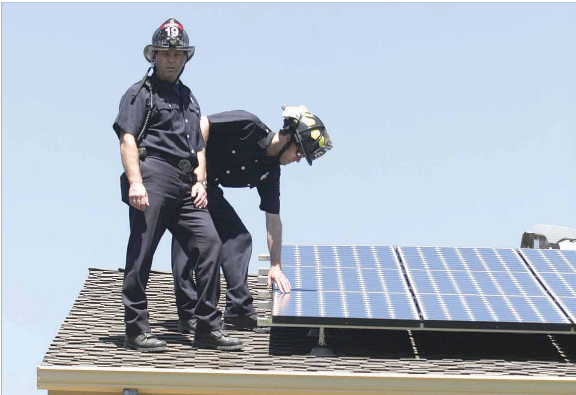
Woodside firefighters Don Bullard, left, and Dave Heckman stand in the 3-foot setback as they inspect a new rooftop photovoltaic system. Solar panels pose challenges and safety concerns to firefighters if a house fire occurs.
