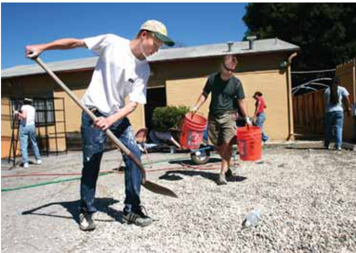
Below: Grant Audet, left, and Brett Hamilton work on a patio at the CityTeam Youth Center in East Palo Alto. Right: Darayn Hickingbotham paints walls at the youth center while Tessa Payne keeps an eye on other volunteers.
