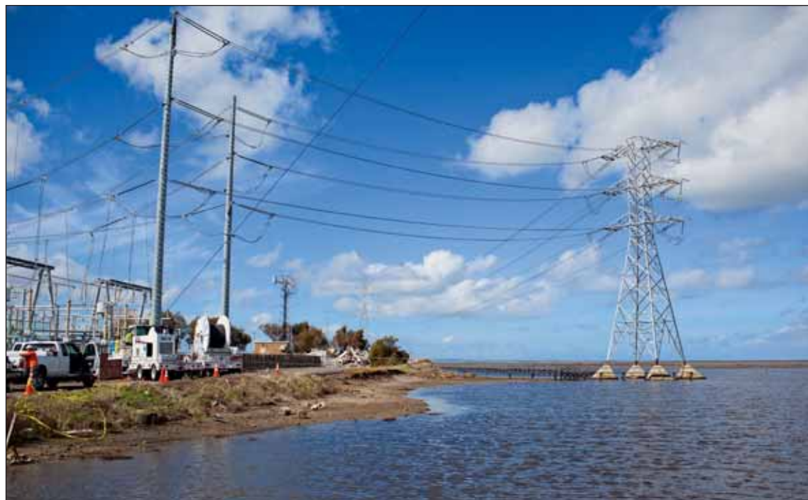
PG&E's Ravenswood Substation is critical to the delivery of power to the Peninsula and a large area in the East Bay. It is at risk from rising sea level.
