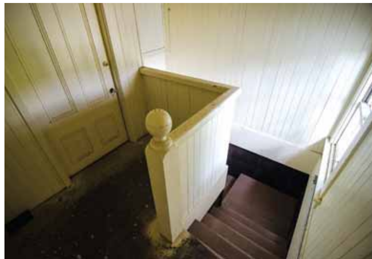
A stairwell leads to the hayloft and the separate space formerly used as living quarters for farmhands.
