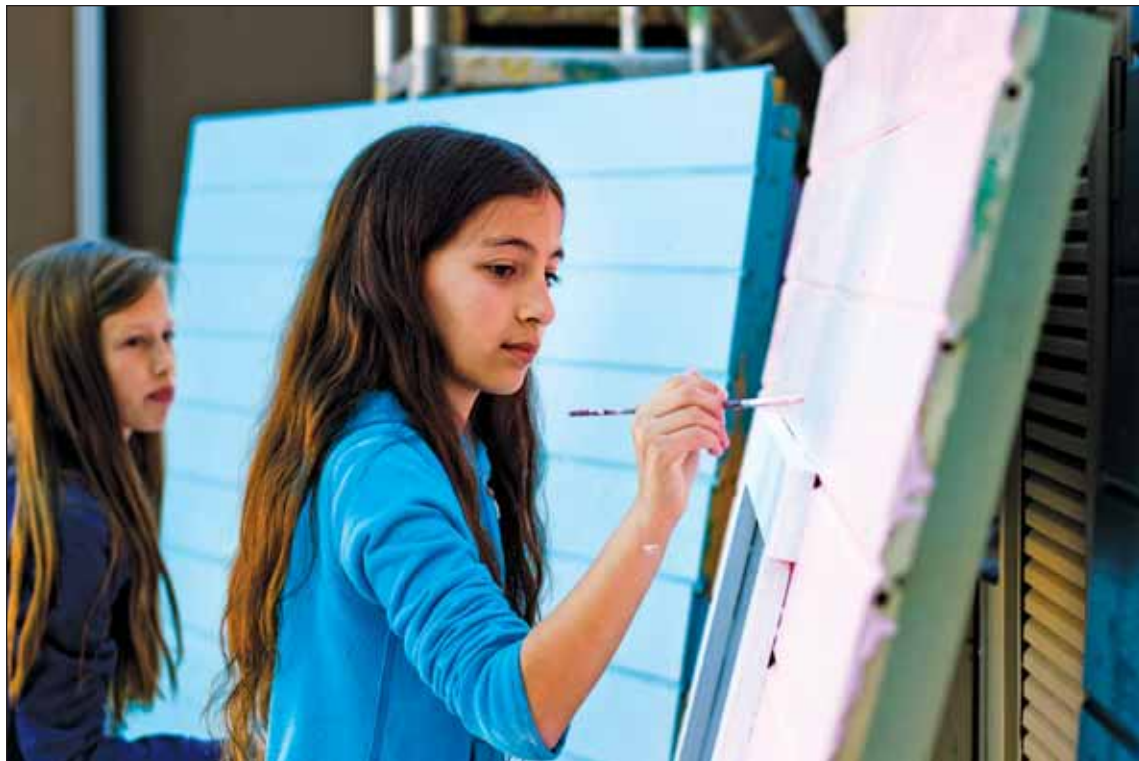
Delaney , 12, adds finishing paint touches to an assembled wall of a playhouse that she and her fellow students built from scratch during the “House That Hillview Built” mini-course.
