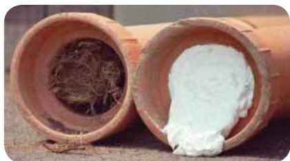
Foam kills and breaks roots, reducing overflows.
