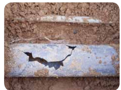
Sewer line repairs can be expensive and not covered by homeowners insurance.
