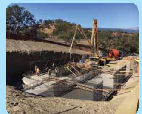
Construction on the District's new Sharon Heights recycled water plant is underway.
