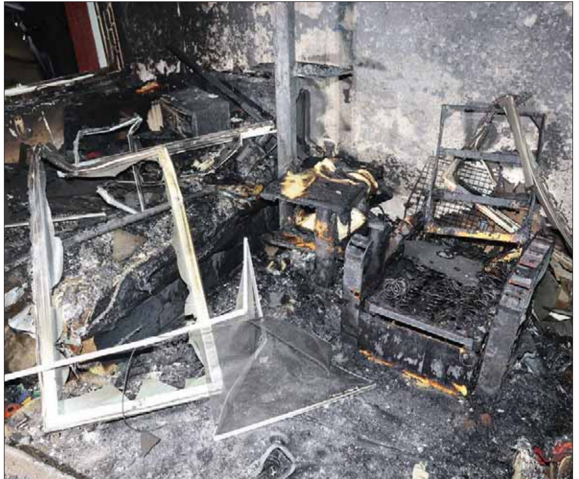
Damage from the fire at 1017 Madera Ave. in Menlo Park on Dec. 24, 2023.
